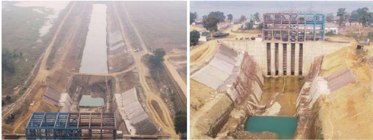
Construction of Check Dam and Water Pump House for Water Conservation, Forebay, Transition Zone and Intake channel, Internal Road & Drain etc, for CW and Make Up Water System
