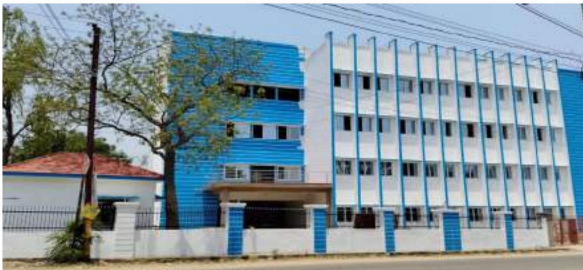
Construction of Commercial office for TP Western Odisha Distribution Limited (TPWODL), Sambalpur (TPWODL is a joint venture between The Tata Power Company Limited and Government of Odisha)
